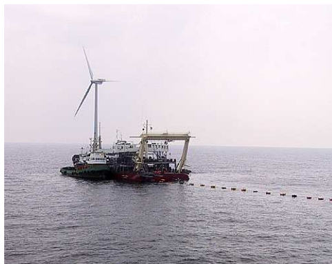
Specialised installation with existing equipment
