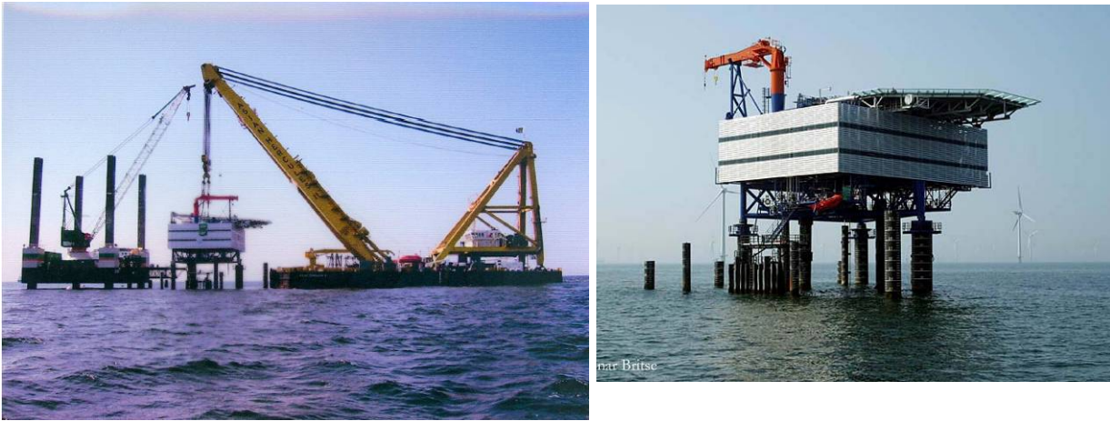
Figure 7-15: Left: “Asian Hercules” delivering the 1200-tonne substation (Source: ELTRA). Right: The ready installed 36 kV to 150 kV substation (Source: Gunnar Britse). The medium voltage cables from the turbines are connected to this substation.
